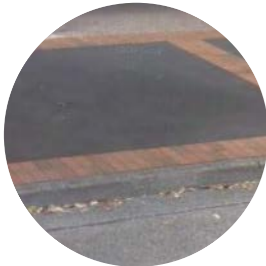
Asphalt & paving bands to secondary street frontages to Council Public Domain controls
